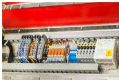
Advanced, PLC based control and DAQ electronics
